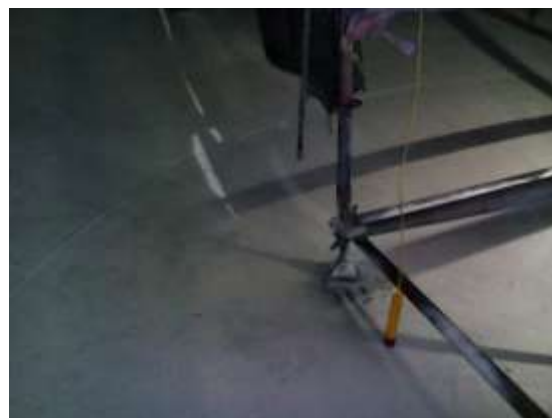
Figure 2. Permanent reference cell #4 (stub) of the bowl area inside the elevated water tank prior to commissioning.
