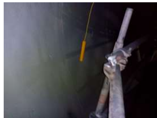
Figure 3. Permanent reference cell #3 near the wall of the bowl area inside the elevated water tank prior to commissioning.
