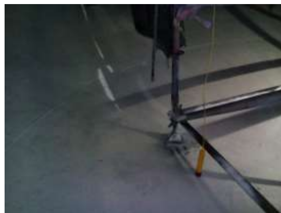
Figure 2. Permanent reference cell #4 (stub) of the bowl area inside the elevated water tank prior to commissioning.
